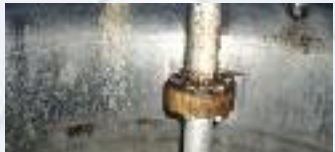
Cleaned tanks after full automatic cleaning procedure.
