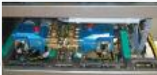
Multiple pump equipment.
