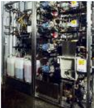
4 pump equipment with different dosing system.
