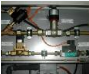
Control and regulation elements of cleaning system.
